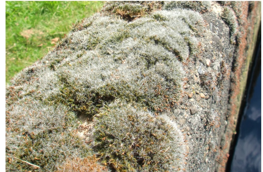
Moss growth and freeze/thaw damage
